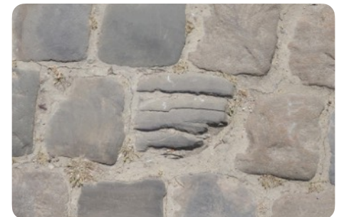
Example of a poorly laid sandstone sett. The cleavage plane must be parallel to the direction of laying. In this case, the sett probably underwent stresses which caused its cleavage. This sett will be discarded during sorting related to reclamation.
